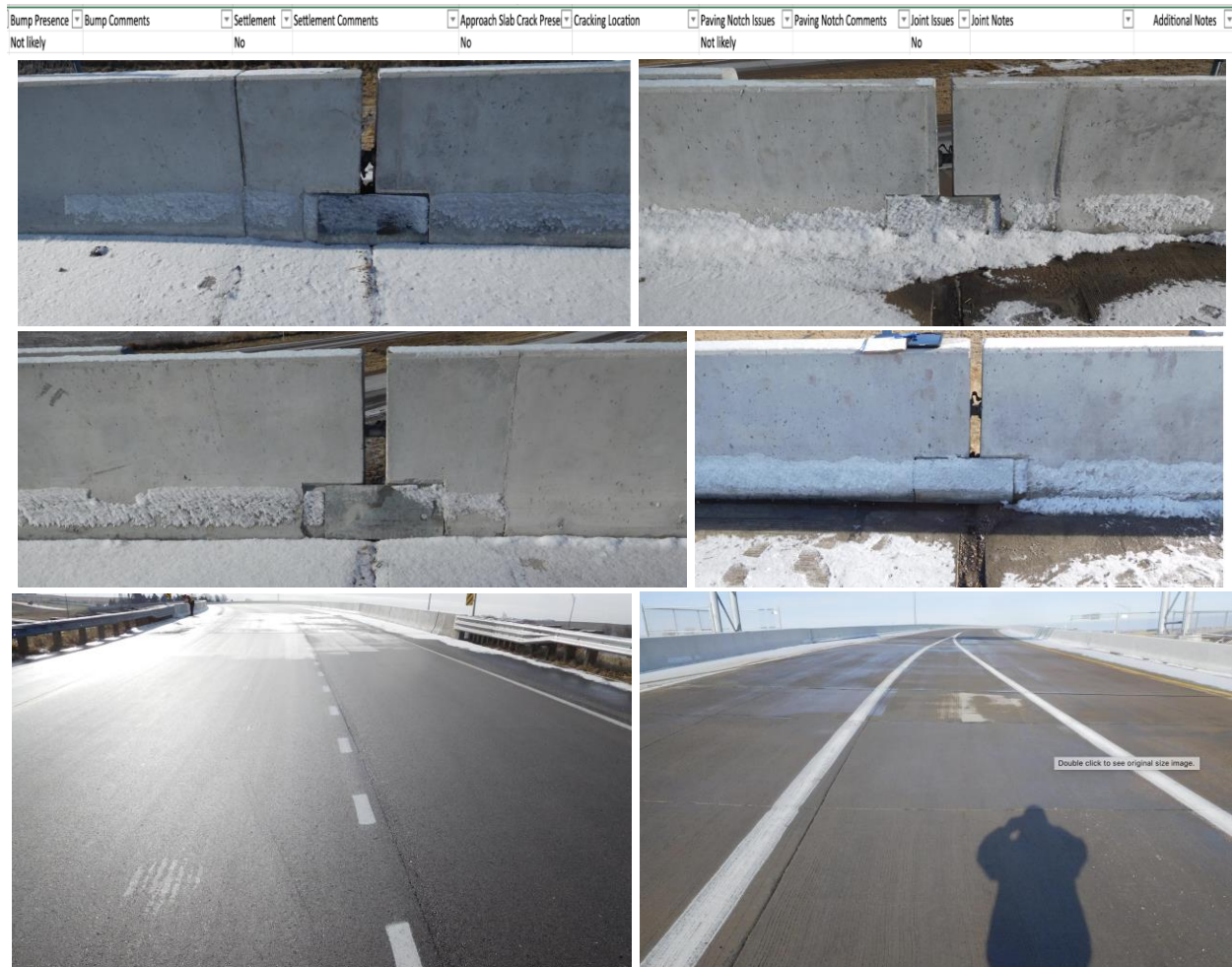
Figure 2.49. Bridge issues table and bridge inspection photographs
