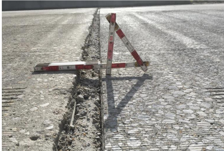
Figure 2.29. Differential settlement at joint
