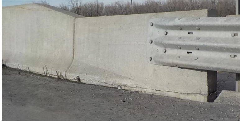
Figure 2.33. Cracking/Differential settlement at barrier
