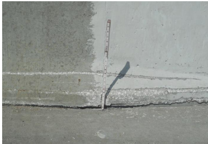
Figure 2.28. Differential settlement at barrier
