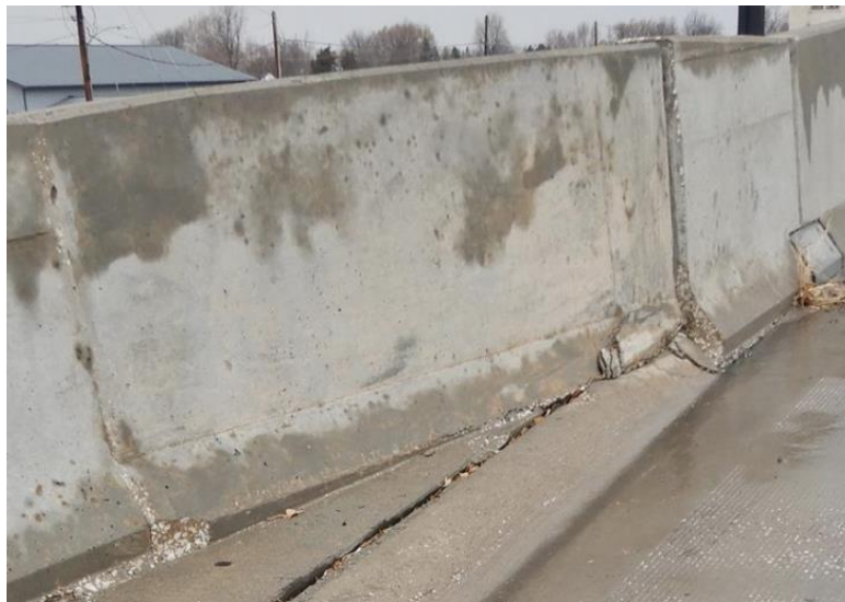
Figure 2.34. Cracking at barrier
