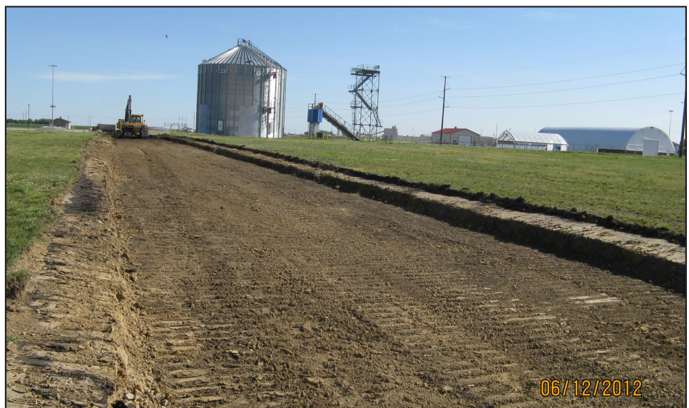
Figure 1. Prepared subgrade prior to placement of PC on the 11th St. North test section
