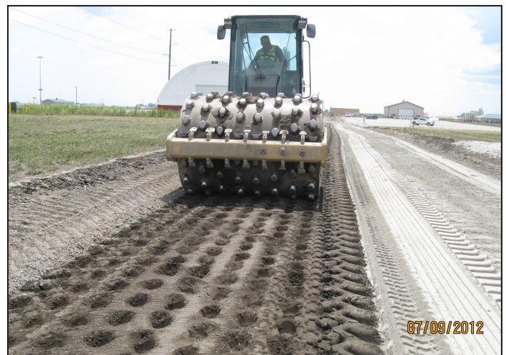
Figure 5. Compaction of a PC-stabilized subbase immediately behind soil reclaimer using a vibratory padfoot roller on 7th St. North
