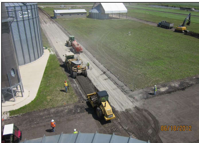
Figure 3. Mixing, moisture-conditioning, and compaction process of PC-stabilized subgrade on 11th St. North
