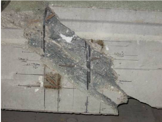
a. shear crack after failure
